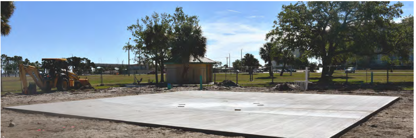
The foundation for the splash pad sits curing in the Florida sun.
