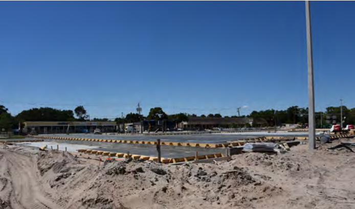
The foundation is poured and walls will soon go up on the Epic Theater.
