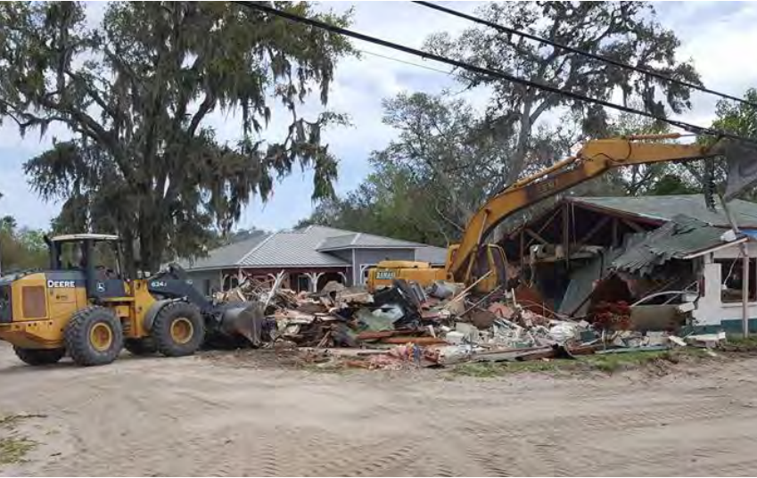
The old Victorio's being demolished in early March, 2016. (Photo: Jason Land / Facebook)
