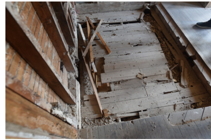
The footprint where a concrete slab and cast iron bathtub once stood on the upper floors of the Old Walker Hotel.
