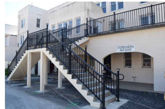
The large, concrete staircase outside the hotel building which will be removed during the renovation.
