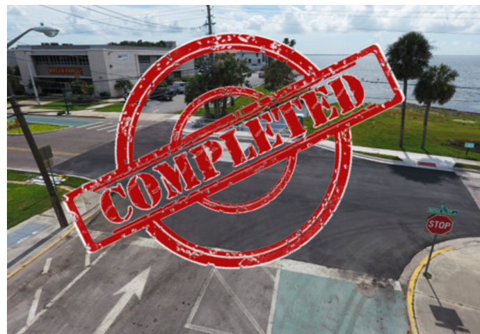
The installation of a baffle box at the intersection of Main Street and Indian River Avenue is now complete, and the road has been reopened.
