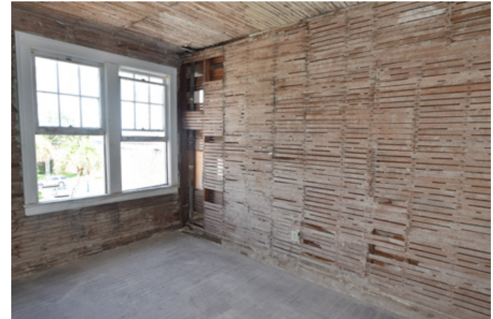
Inside one of the many rooms on the upper floors of the old hotel that will be renovated into boutique-style apartments.
