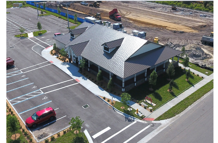
Construction is nearing completion for a 6,600-square-foot restaurant located along Helen Hauser Boulevard, south of S.R. 50.
