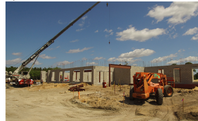
Site construction continues on a 119-unit hotel and a 2-story office/retail building at the corner of U.S. 1 and Riverfront Center Boulevard (formerly Vectorspace Boulevard).
