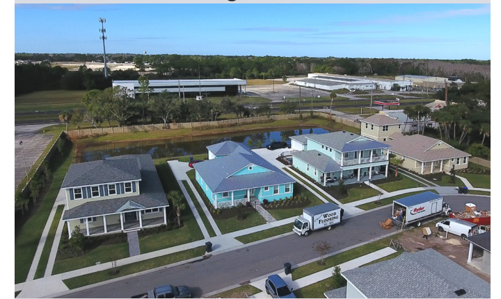
Several homes have been completed and more homes are under construction at the 22-lot subdivision located on Riveredge Drive.
