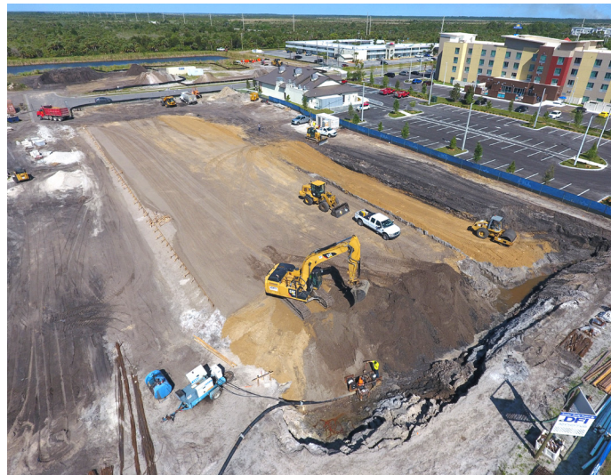
Construction has begun on a 124-unity, 4-story hotel located at the southern terminus of Helen Hauser Boulevard adjacent to the new Durango's restaurant.
