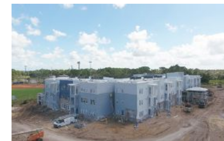
Site and building construction continues on an 84-unit, three-story apartment complex located at the southeast corner of Sycamore Street and Deleon Avenue.
