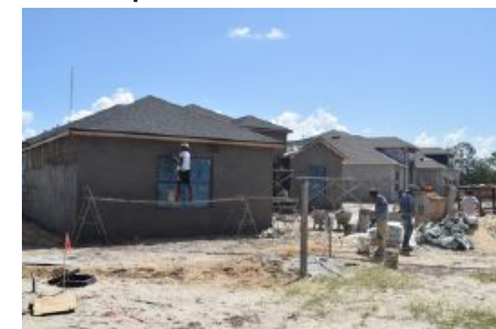
Site construction continues and several homes are under construction for a 70-lot, single-family home subdivision located west of I-95, north of Fox Lake Road.
