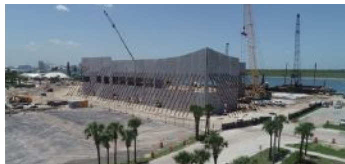
Cruise terminal construction underway at Port Canaveral. (Image courtesy of Canaveral Port Authority)
