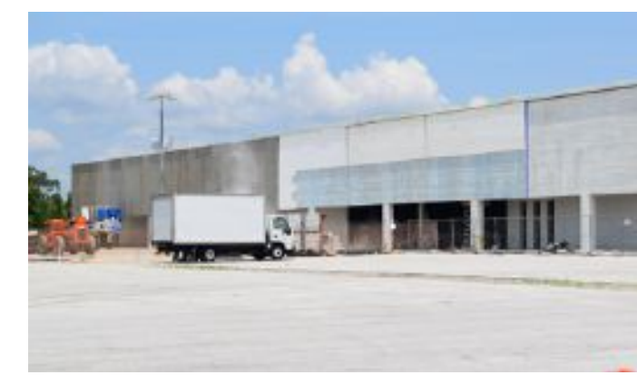
Site construction is underway to redevelop the former Kmart building into indoor, climate controlled storage located at 810 Cheney Highway.
