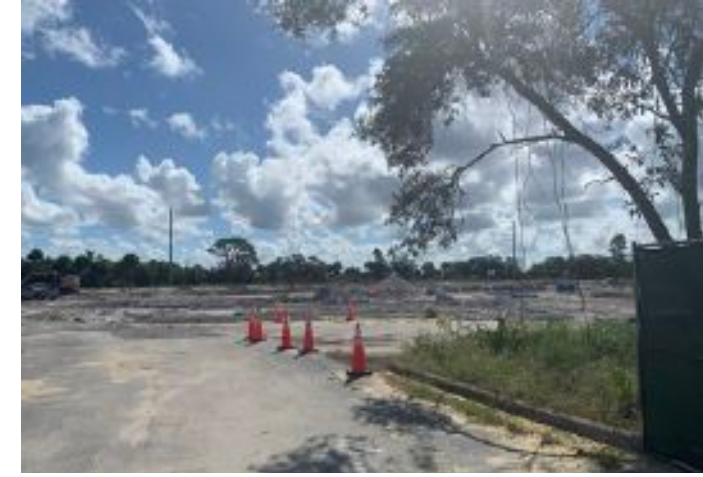
Site construction continues for a 152-room, five-story hotel with an observation deck to be located at 6225 Riverfront Center Boulevard, on the property of the former U.S. Astronaut Hall of Fame. The hotel will be operated by Delaware North, who also operates Kennedy Space Center Visitor Complex, and will include 800 square feet of meeting space for conferences and special events.
