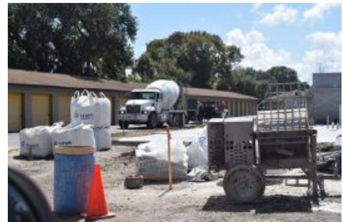
Site construction is underway for an expansion of the existing storage business located at 1903 Garden Street. The scope of work includes the demolition of two existing one-story buildings and construction of one three-story building to be comprised of indoor storage units.
