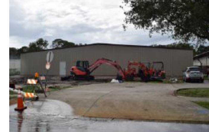
Site construction continues for a 10,000-square-foot addition to the existing building located at 411 S. Park Avenue. Aero Electronics Systems is a Defense Department contractor which specializes in manufacturing cable assemblies as well as braided and molded cables for use in military applications such as torpedoes, missiles, and aircraft. (Article on page 7)
