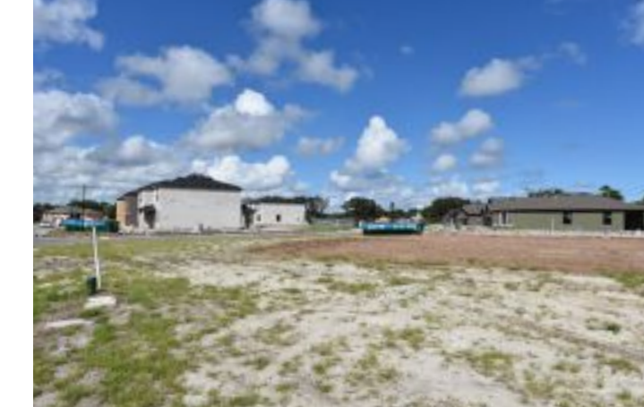
Site construction continues and several homes are under construction for a 39-lot, single-family home subdivision located at the southeast corner of Knox McRae Drive and S. Park Avenue.
