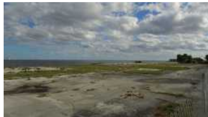
Site work began on River Palms, consisting of two condo buildings totaling 100 residential units at 1805 Riverside Drive across from Titusville High School.
