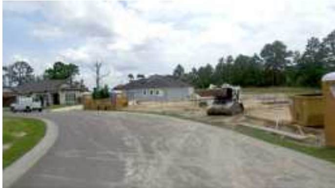
Site clearing began for South Carpenter Estates in 2018, beginning construction of 70 single family homes on South Carpenter Road near the corner of Fox Lake Road.
