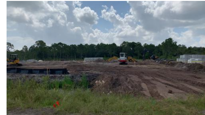
Site construction continues for a 13,400-square-foot office and fabrication shop/warehouse at 1825 Shepard Drive.
