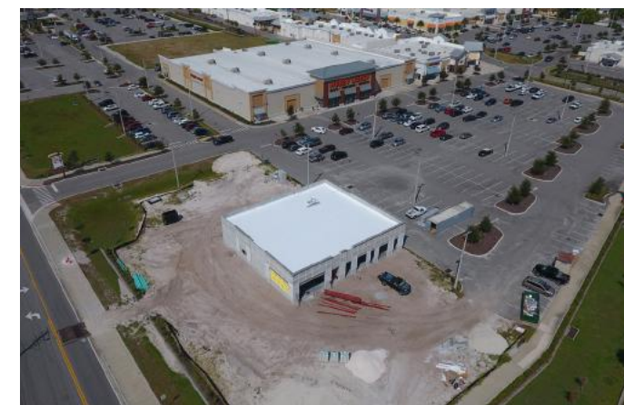
Site and building construction continues for a 6,475-square-foot restaurant building consisting of a 2,400-square-foot Chipotle, and another 3,750-square-foot restaurant space, located at 2560 South Washington Avenue.
