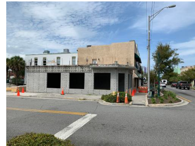
Site and building construction continues for a 2,316-square-foot office building located at 346 S. Washington Avenue
