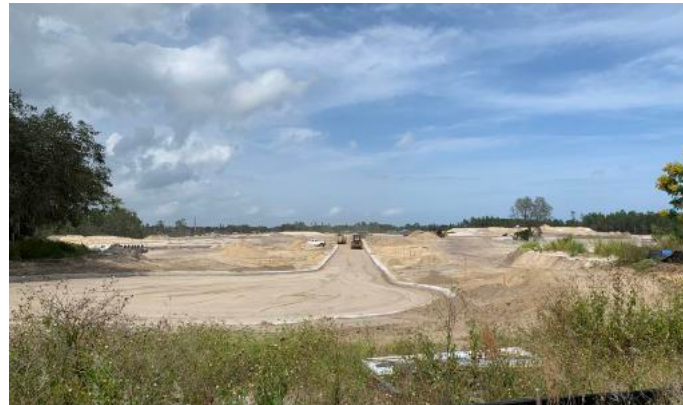
Site construction continues for a 166-lot single-family home subdivision located north of Garden Street, east of N. Carpenter Avenue.
