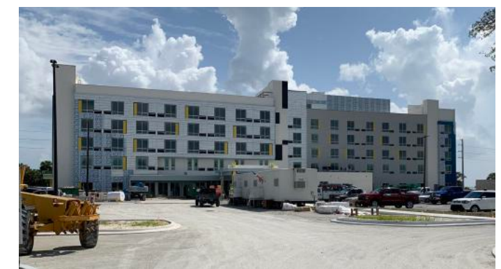
Construction continues on the 152-room, five-story hotel that will also feature a rocket launch observation deck on the roof. The new hotel is located adjacent to the Lockheed Martin STAR Center (former US Astronaut Hall of Fame).
