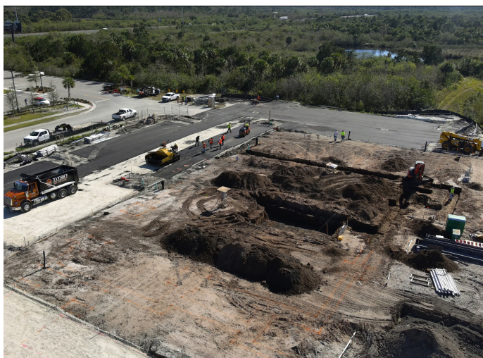
Site construction continues on a 68,992-square-foot, 122-room hotel located at 4830 Helen Hauser Boulevard.
