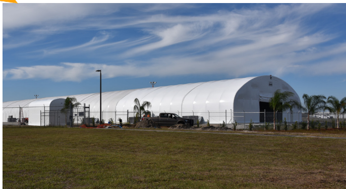
Site construction continues for a 49,000-square-foot manufacturing building located on Bristow Way at the Space Coast Regional Airport.
