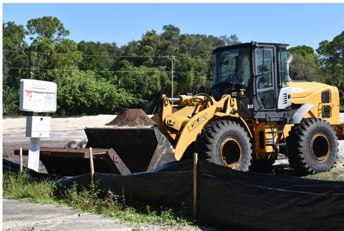
Site construction continues for 28 two-story townhome units located south of E. Whispering Hills Road and east of Elizabeth Avenue.
