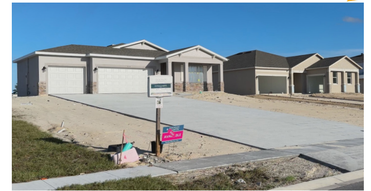
Site construction is complete and single-family home construction is underway for a 170-lot subdivision found at the northwest corner of Garden Street and I-95.
