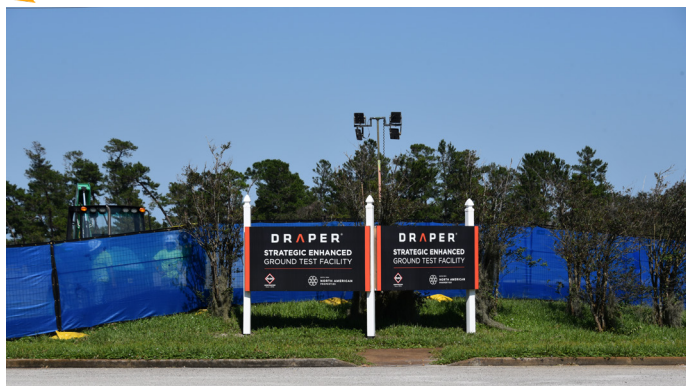
Site construction is underway for a 50,920-square-foot laboratory building located at 6280 Riverfront Center Boulevard.
