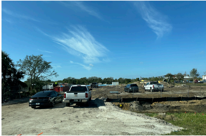
Site construction is underway for a 51,470-square-foot self-storage building, as well as covered outdoor RV storage.
