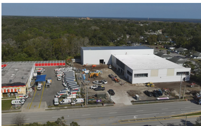
Construction continues on a 16,157-square-foot warehouse and 44,238-square-foot self-storage building at 2060 Garden St.
